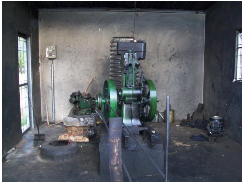
Figure 33- Crudely repaired main pump in Skoonheid
