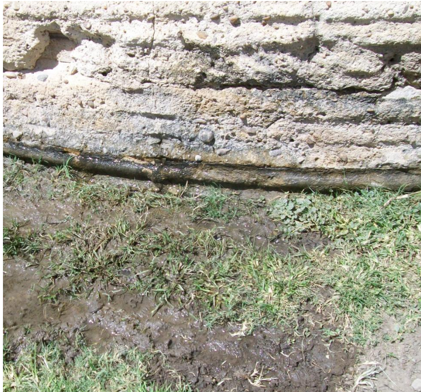
Figure 34- Leaking dam in Skoonheid
