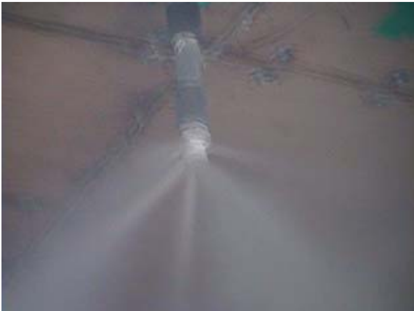
Photograph 6. CO2 Discharge into Enclosure
