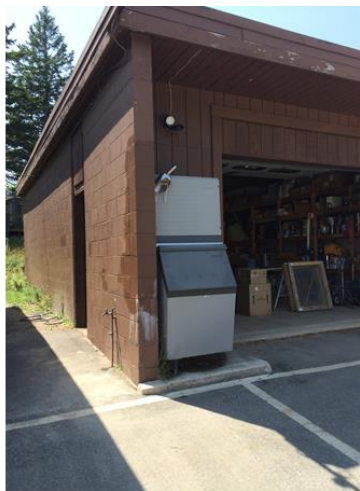
Figure 10: Ice Maker at the HQ Garage
