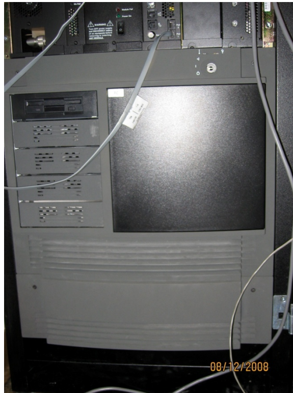
Figure 15: Radio Network Controller (RNC)
