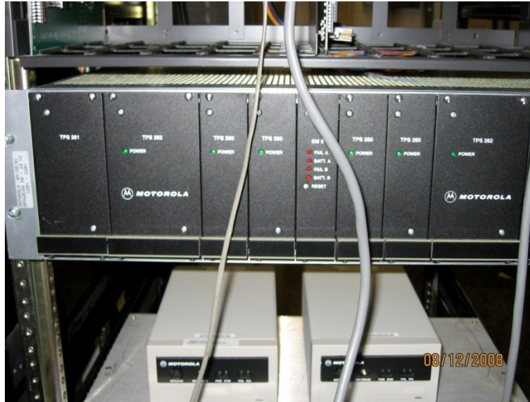
Figure 8: Centracom Gold Power Supply
