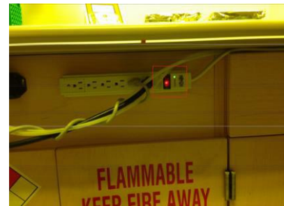
Figure 6: Hot Plate Power Strip
