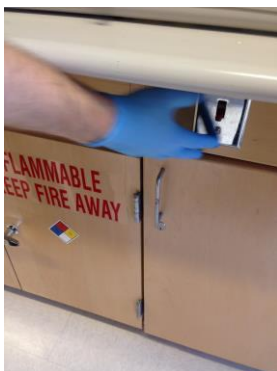
Figure 5A: Vacuum Pump Switch
