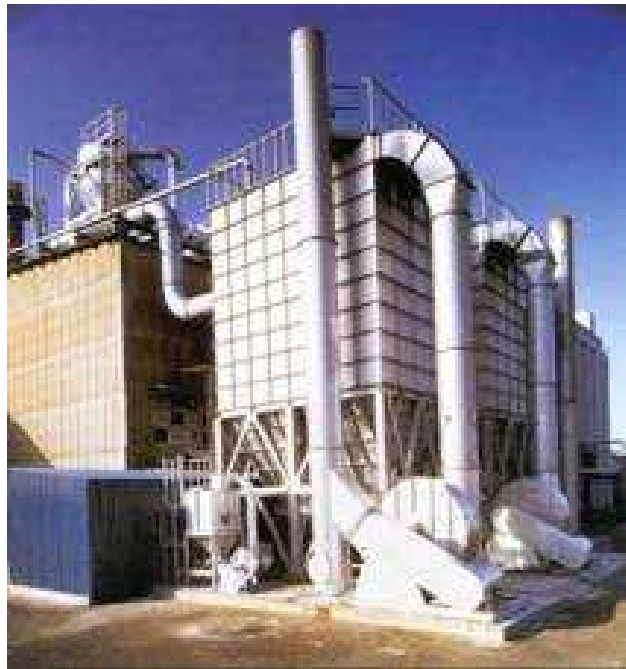
Figure 38: Flue Gas Dry FGD System
