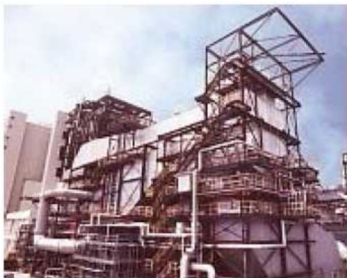
Figure 45: FGD at Lamma power station
