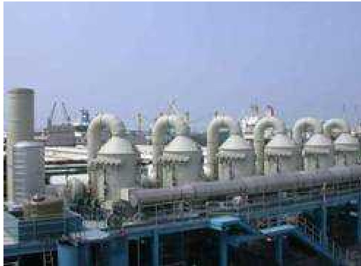
Figure 36: Wet Scrubbers & Ventilation System
