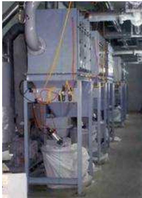
Figure 35: Central vacuum dust collector
