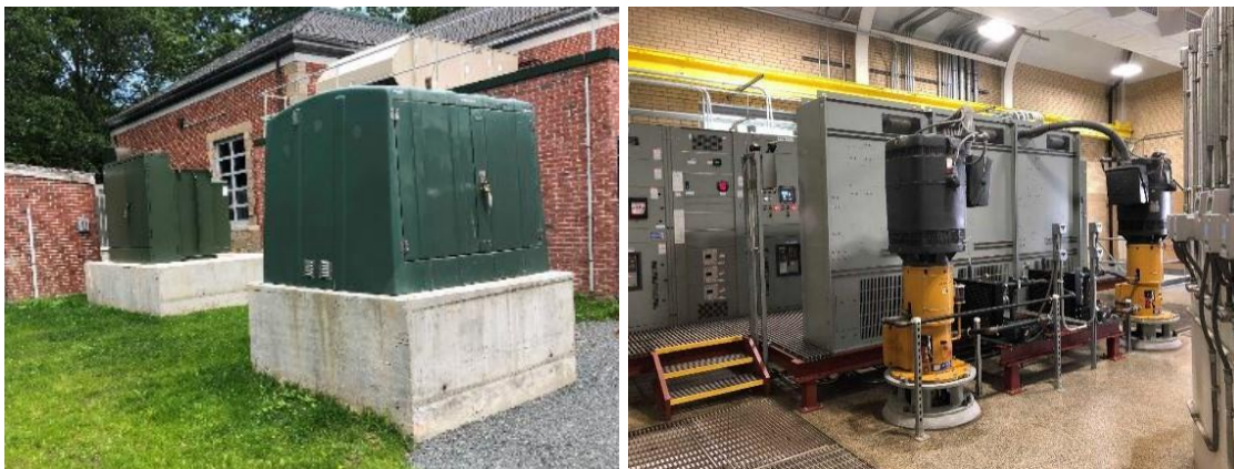
Figure 5 (left): Alewife Brook Pump Station Raised Outdoor Equipment
