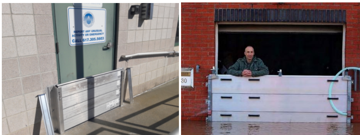
Figure 4.6 (left): Doorway stop log protects facilities from potential flooding (MWRA - How MWRA Is Preparing for Climate Change, n.d.)
