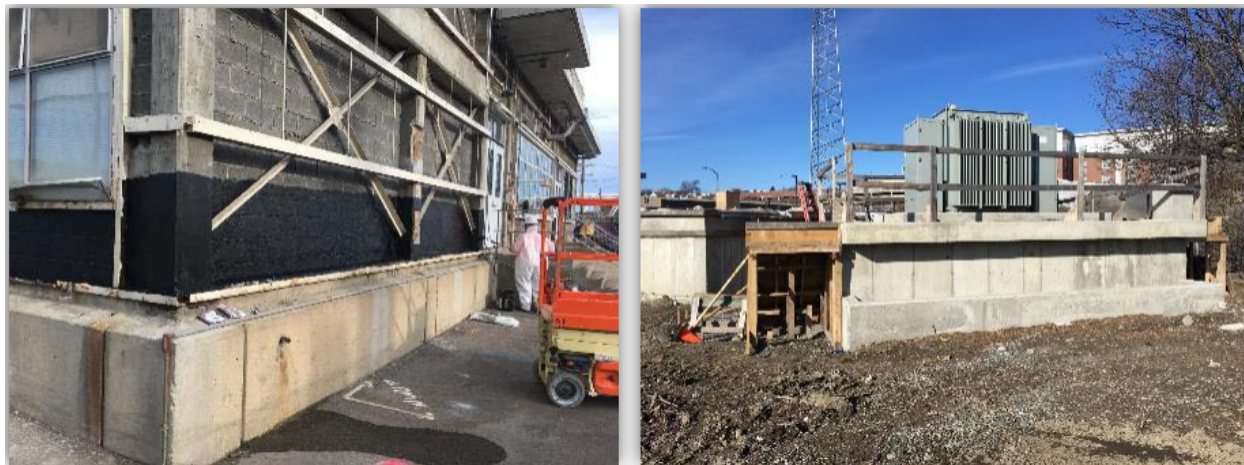
Figure 4.5: Chelsea Headworks reinforced elevated foundations and flood protection (Climate Resiliency At MWRA (PDF), 2019)
