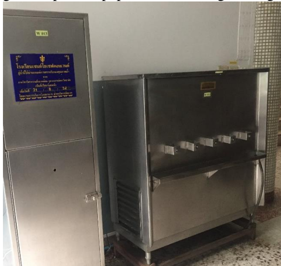
Figure 4.4: Water Filter at SJC
