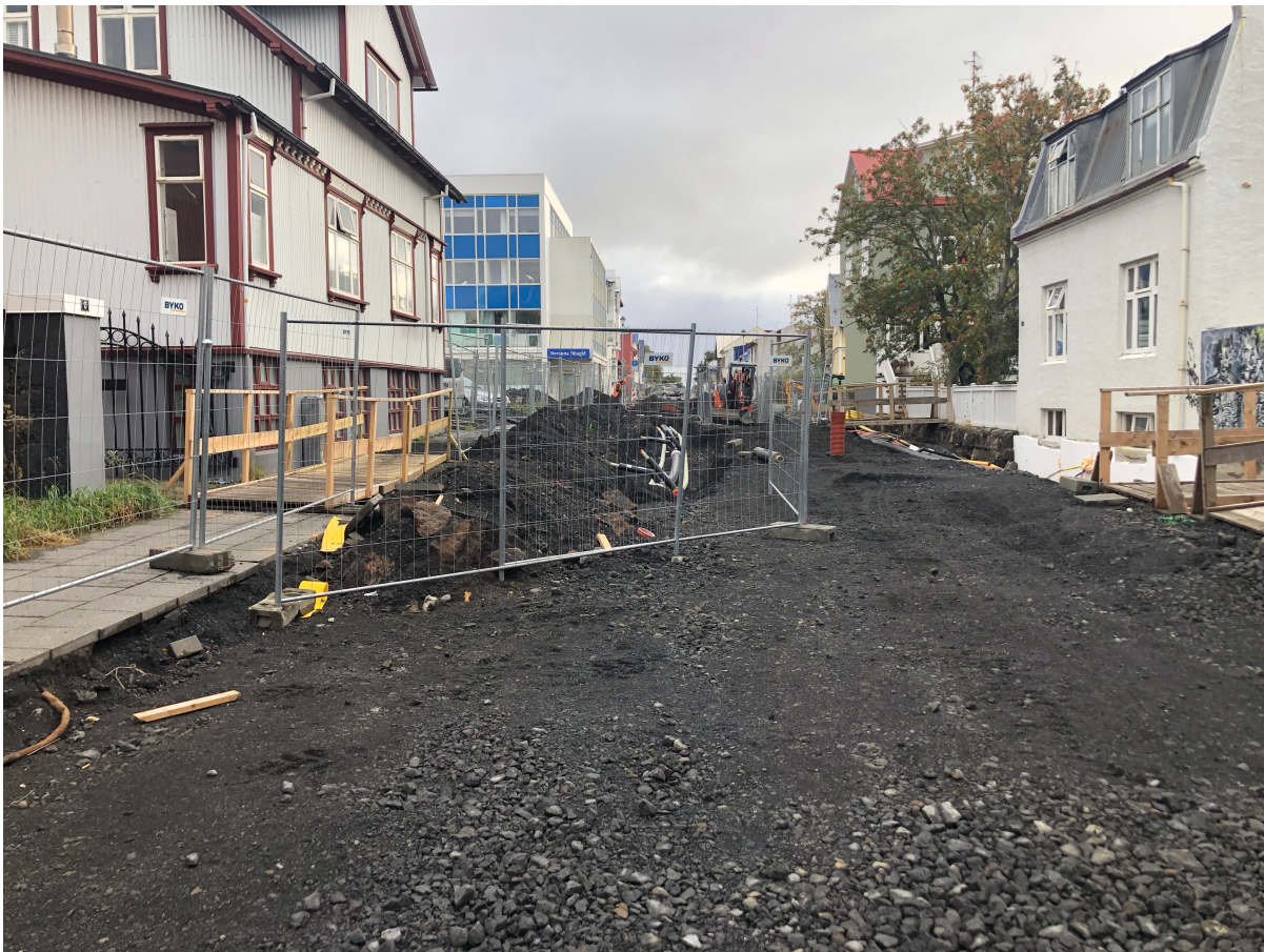
Figure 8. Road construction on Tysgata disrupting traffic patterns and reducing CBD parking (fall 2019).
