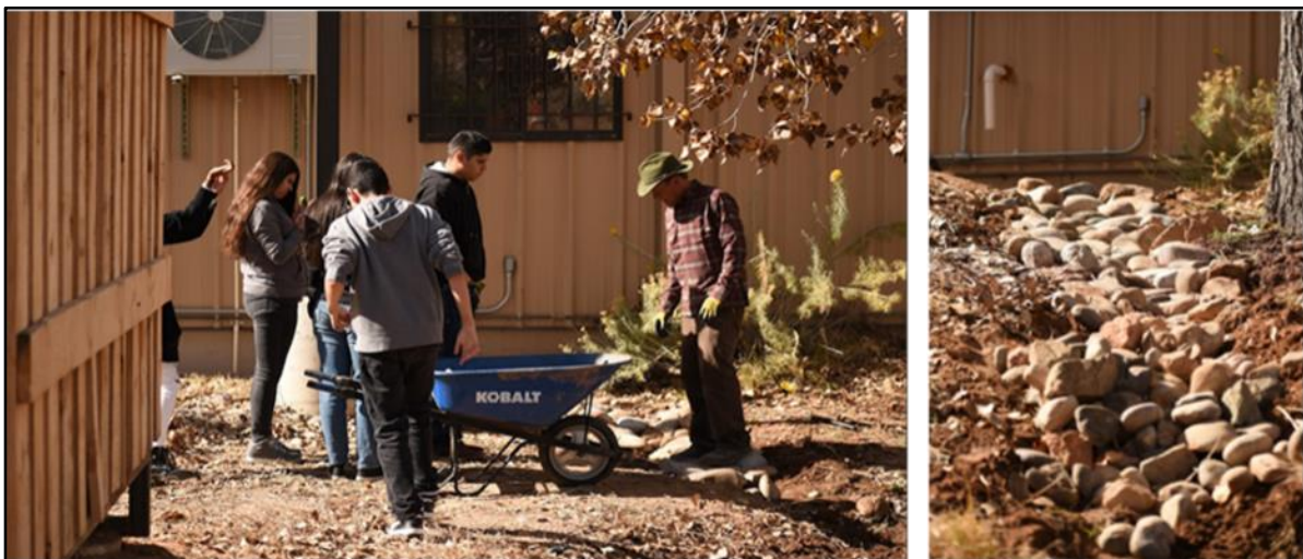
Figure 12: Pictures show Rich working with the kids collecting rocks to build the erosion control dam pictured on the right.
