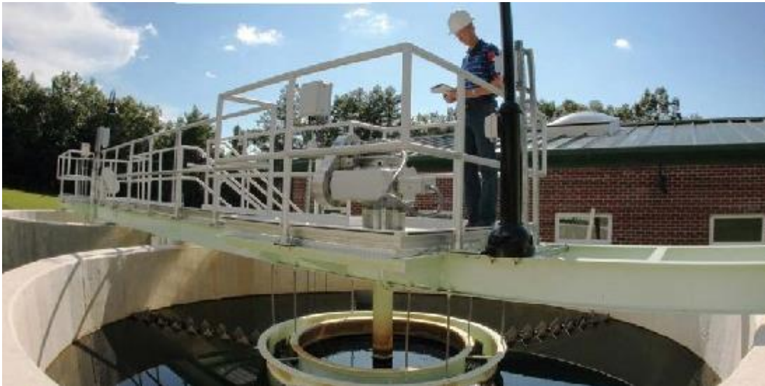
Figure 8: CoMag® system at a 2.2 MGD WWTP
