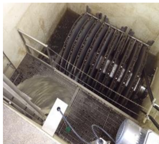
Figure 4: AquaDisk® Cloth Media Filtration System at the Portland, Indiana WWTP
