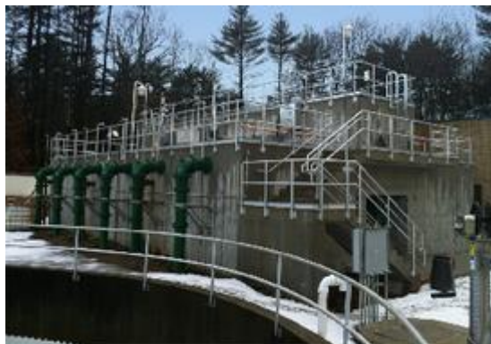
Figure 5: Blue PRO® System at the Westerly, MA WWTF
