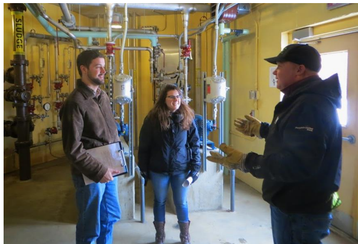
Figure 14: Operator Bob Fischer giving the MQP team a tour of the facility
