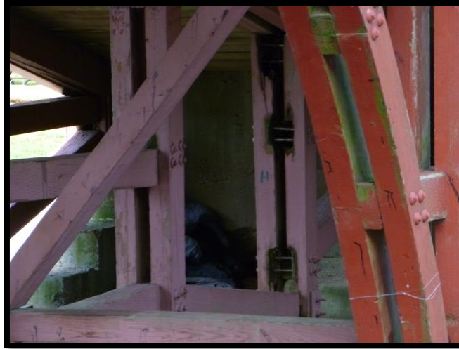
Figure 13: Example of previous bridge structure deficiencies - missing beams.
