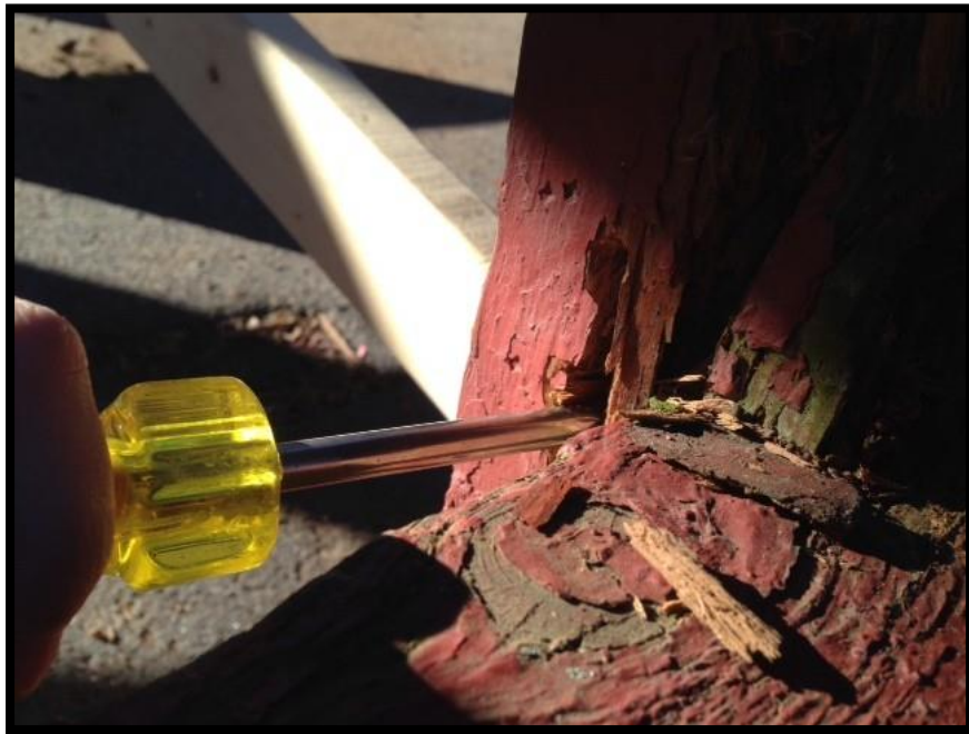
Figure 88: Pick test result indicating decayed wood
