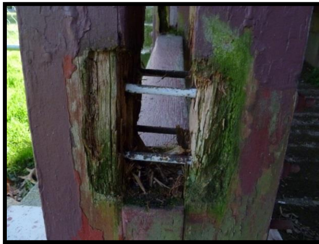
Figure 14: Example of previous bridge structure deficiencies - rotting connections.
