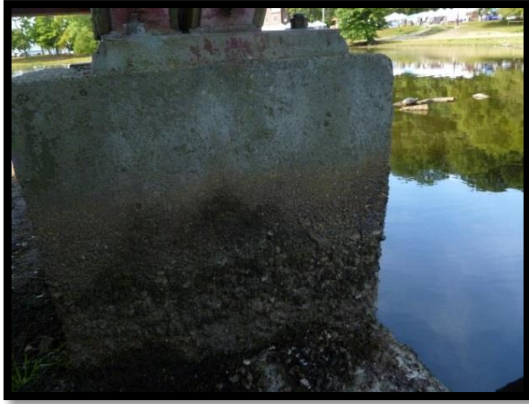
Figure 64: Image of current bridge footings - close up view of a single pier.
