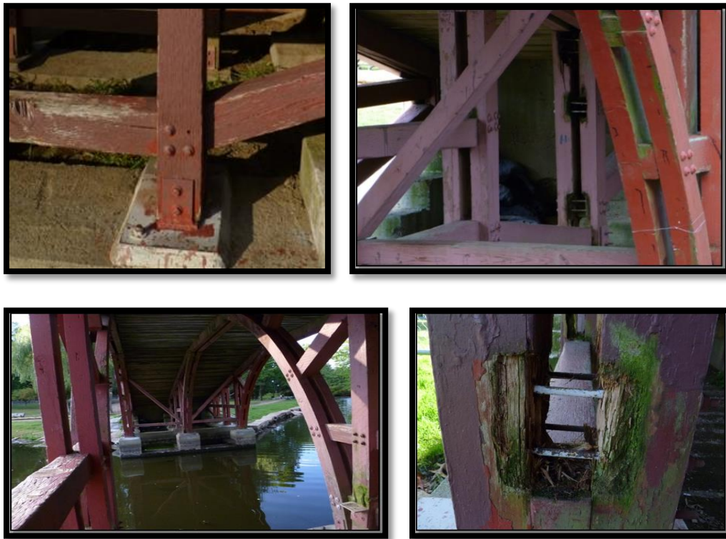
Figure 85a, b, c, and d: Images of bridge's failure points. Top Left: missing bolts. Top right: missing beams. Bottom left: missing cross-bracing. Bottom right: rotting connections.
