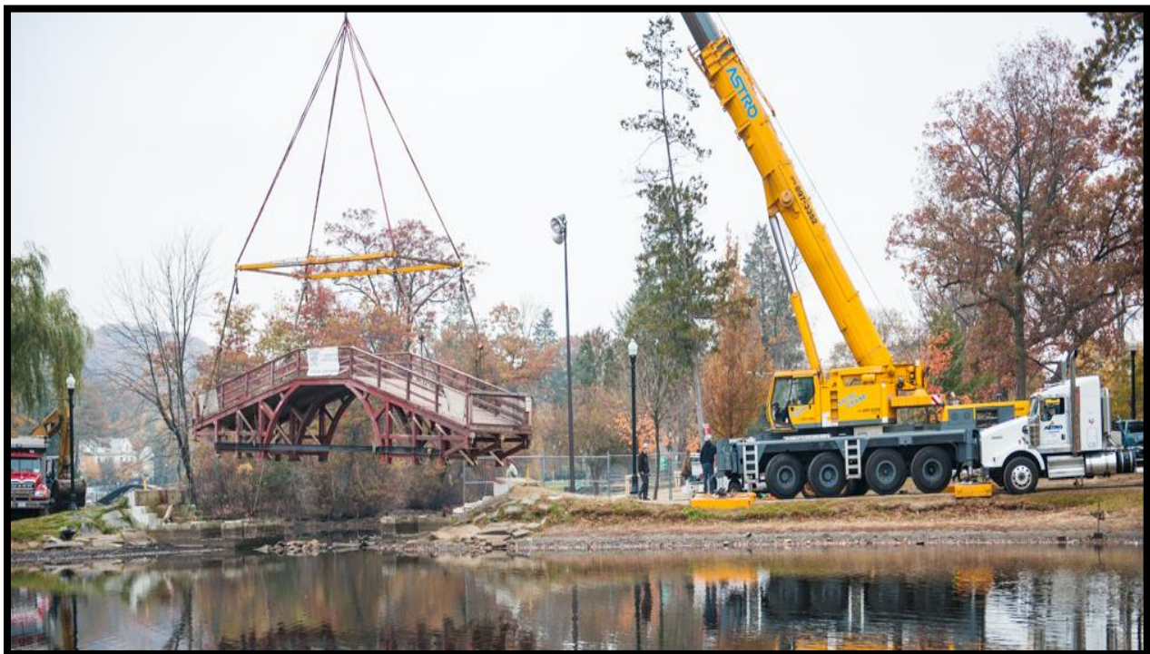
Figure 20: Image of the Elm Park Bridge being removed from Elm Park. Source: (Worcester Magazine, 2013)
