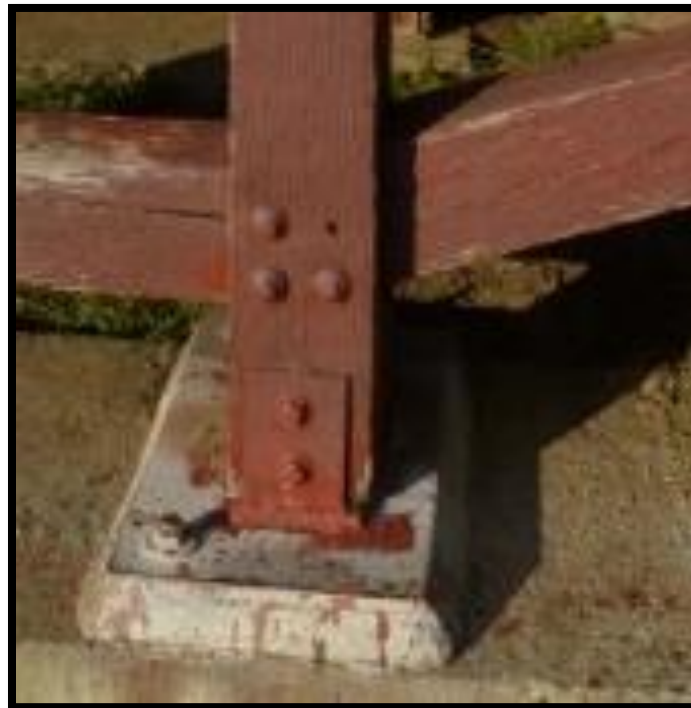
Figure 12: Example of previous bridge structure deficiencies - missing bolts.
