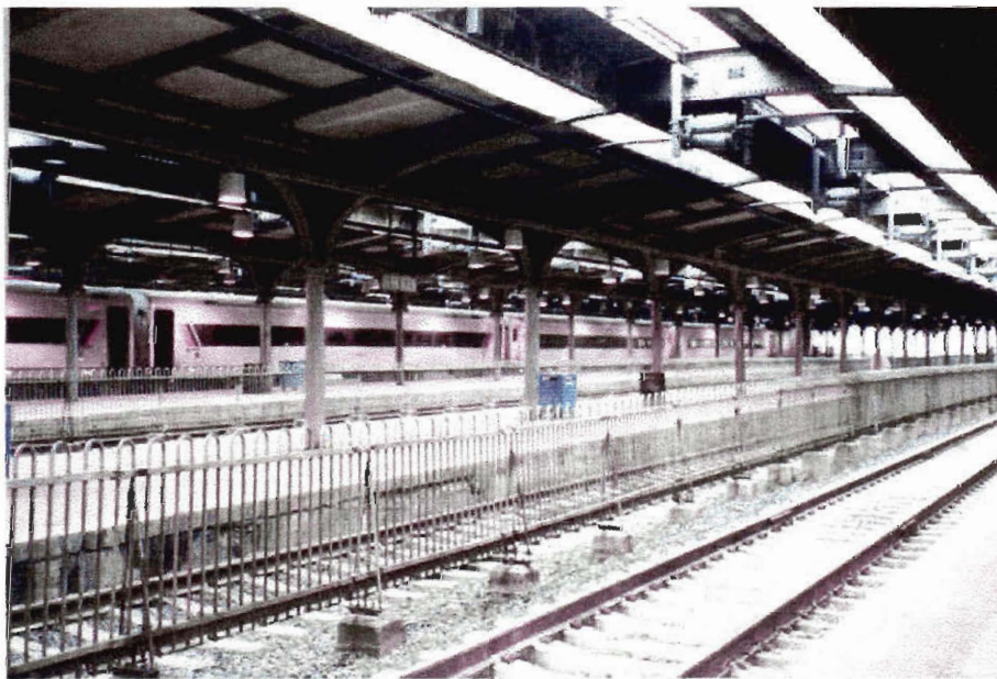
Figure 2-2 A New York Train Station-Evidence of New York's Application of the Broken Windows Theory
