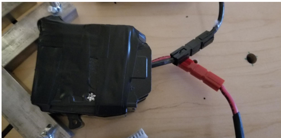
Figure 41: 60 amp breaker attached to LiPo cells
