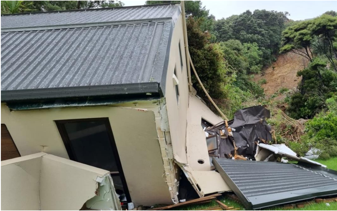
Figure 1. A house in West Auckland collapsed after a slip
