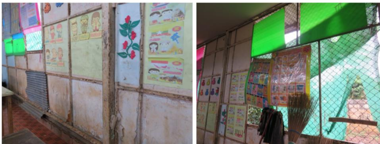
Figure 3: Conditions inside third grade classroom. The photo on the left shows the deterioration of the walls and the photo on the right shows the chain-linked windows.
