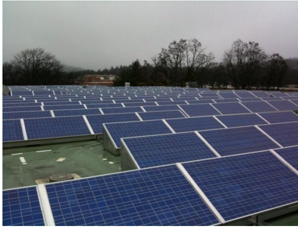
Figure 11 WSC Solar Array Front View (Collins, 2009)
