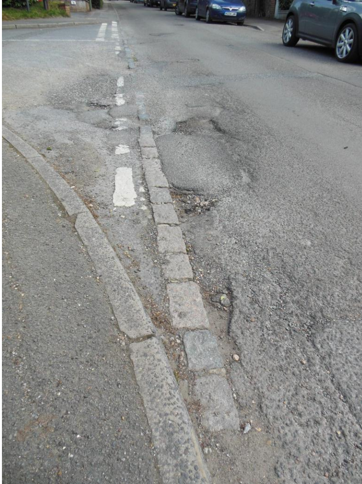
Figure 17: Series of potholes on Doods Road
