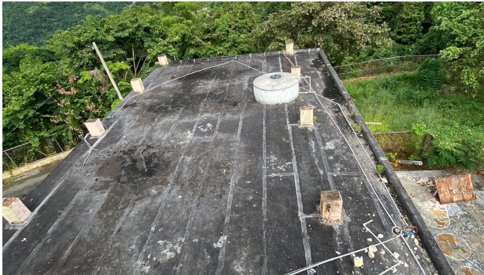
Image 6: Example of blistered and cracked roof at the Cubuy Community Center
