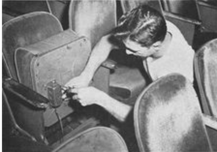
The electrician above, is shown installing one of the Percepto units underneath the theatre seat.
