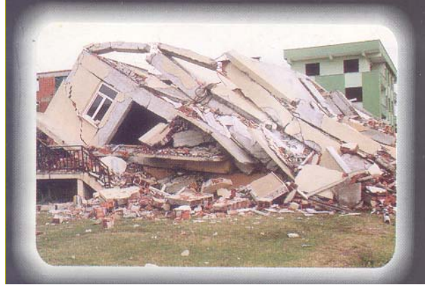
Figure 3-18 The earthquake insurance will hopefully cover the unexpected building damages resulted by earthquakes
