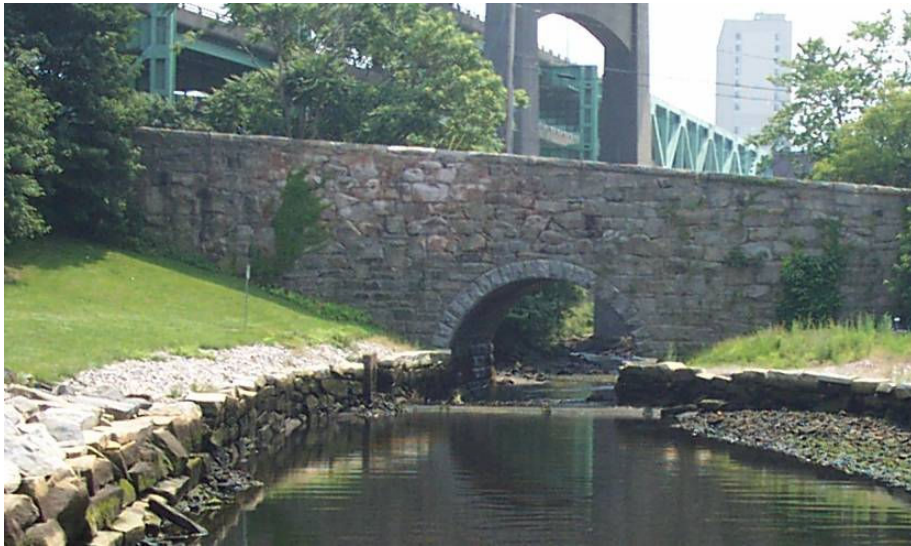
Figure 1. Photo of North Elevation of the Central St. Bridge. Photo by Author.
