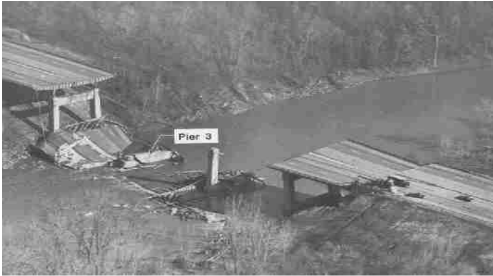
Figure 12. Photo of Schohaire Creek Bridge April 5, 1987. Courtesy of the National Bridge Inventory Web Page.
