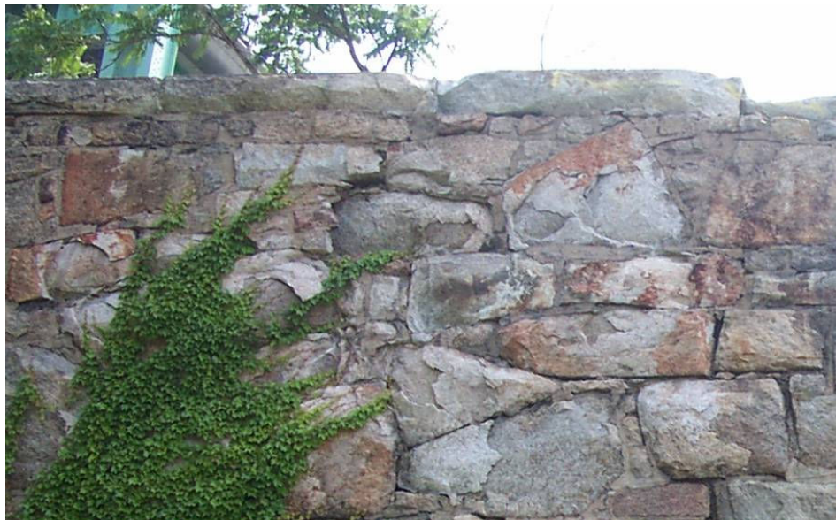
Figure 2. Photo of North Spandrel Wall Damage. Photo by Author.
