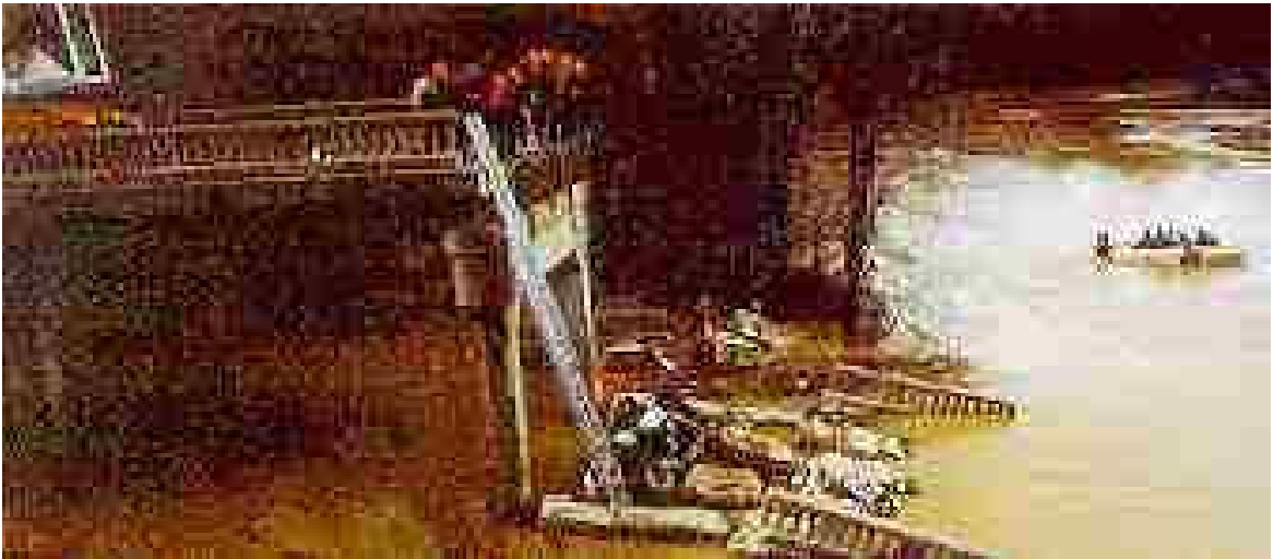
Figure 13. Photo of U.S. Route 51 Bridge Collapse. Reprinted from The Turner Fairbanks Research Center News Letter 59.1 (1995).
