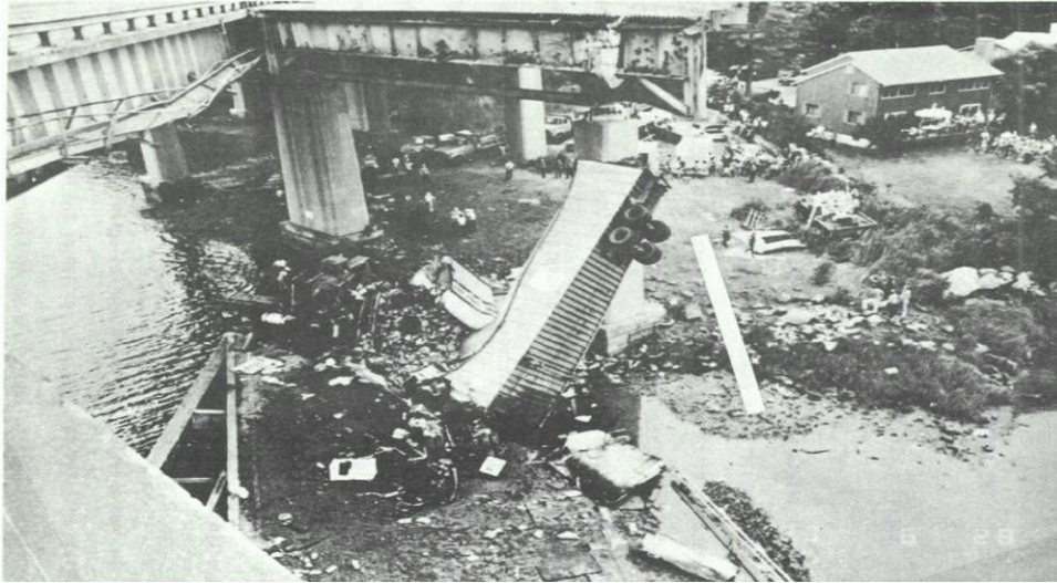
Figure 10. NTSB photo of Span 20 eastbound, Mianus River Bridge. Reprinted from USDOT, Inspection of Fracture Critical Bridge Members , (Washington, D.C. 1986), 2.
