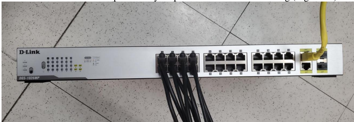
Figure 47: Switch Box with Camera Inputs and PC Outputs
