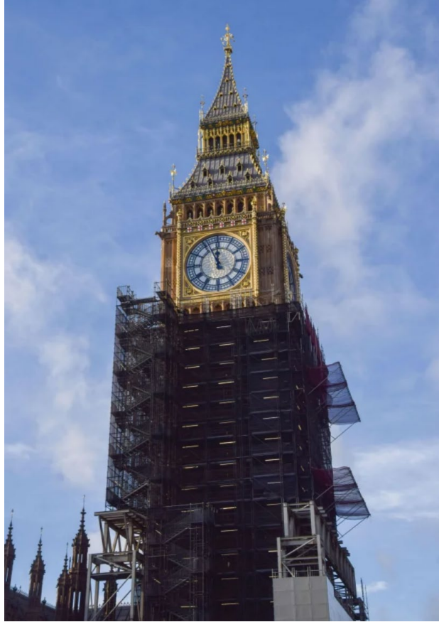
Figure 33. A recent restoration of London's iconic Big Ben clock tower. Source: URL .
