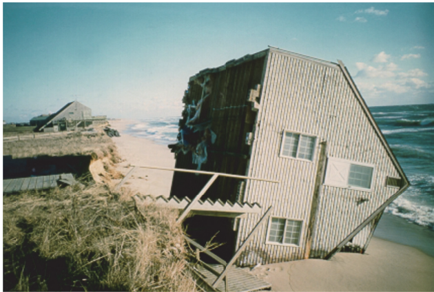
Figure 2: Bluff erosion under a home on Nantucket (Photo by Stephen P. Leatherman, 1996)
