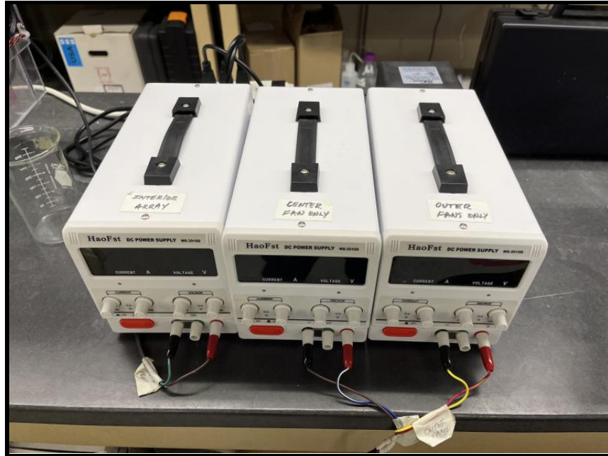
Figure 10: Power Supply Boxes
