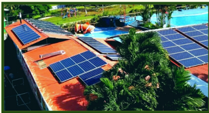
Figure 3: Solar Panels Installed on a roof
