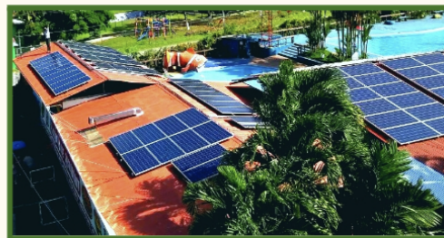
Figure 2: Solar Panels Installed on a roof
