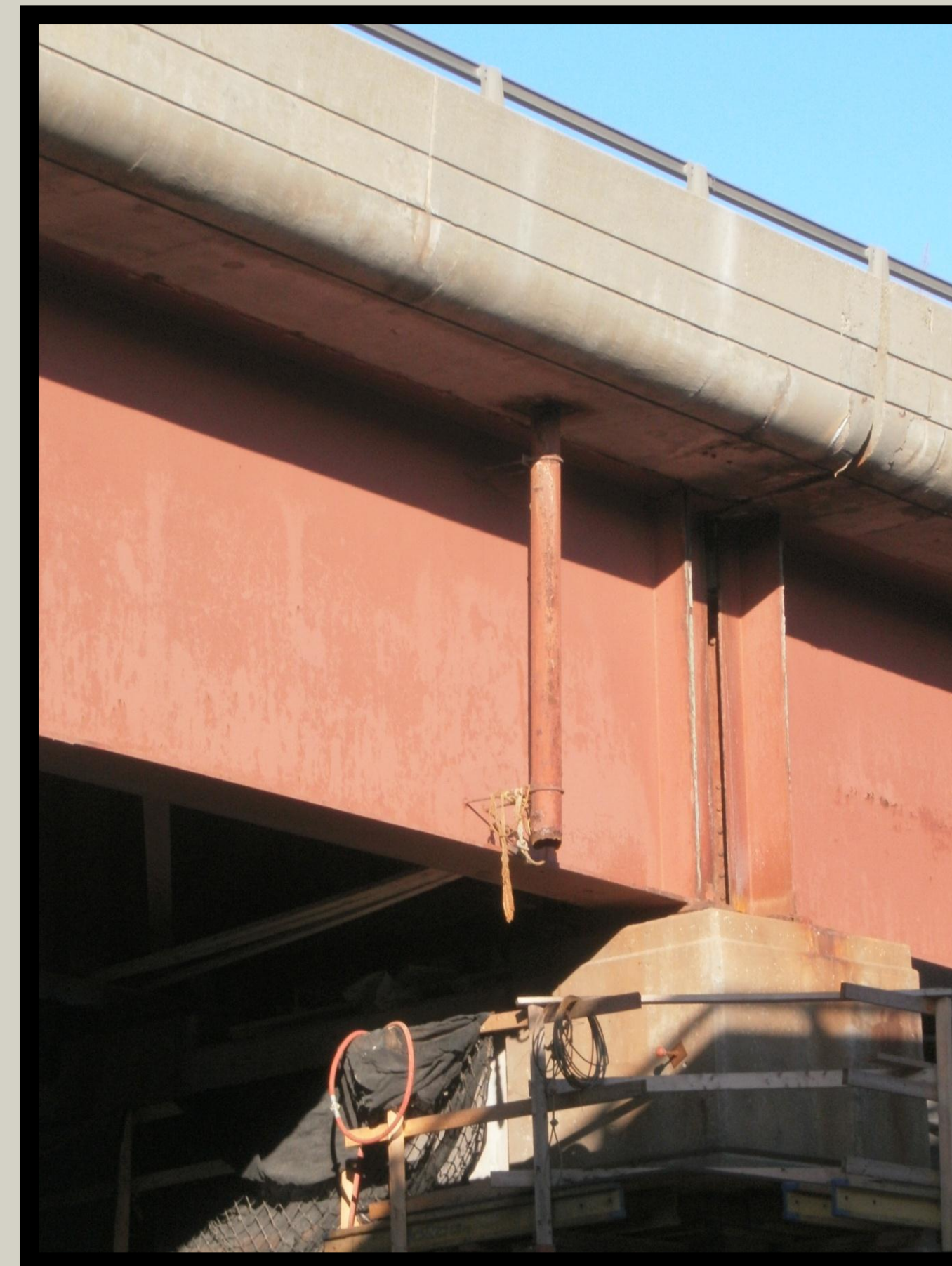
Drainage Pipe off the I-290 bridge over Lake Quinsigamond. © UWM Groups
