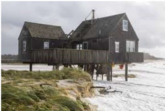
Figure 16: Former Stilt house built near Millie's Bridge (Nicole Harnishfeger. (Mar 2018). "Stilt House." Inquirer & Mirror )
