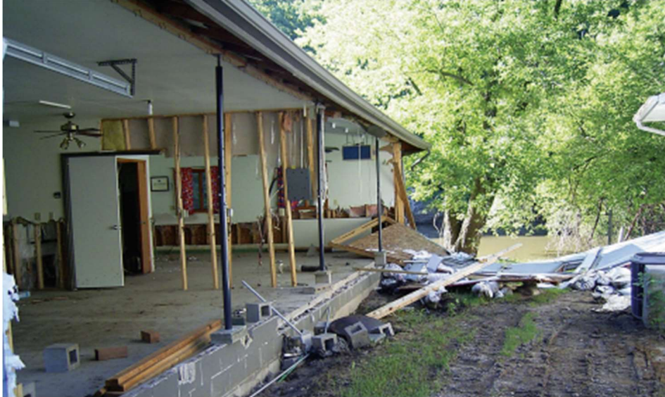
Figure 14: A home which had the wall ripped off due to flood water velocity (FEMA, p.31)
