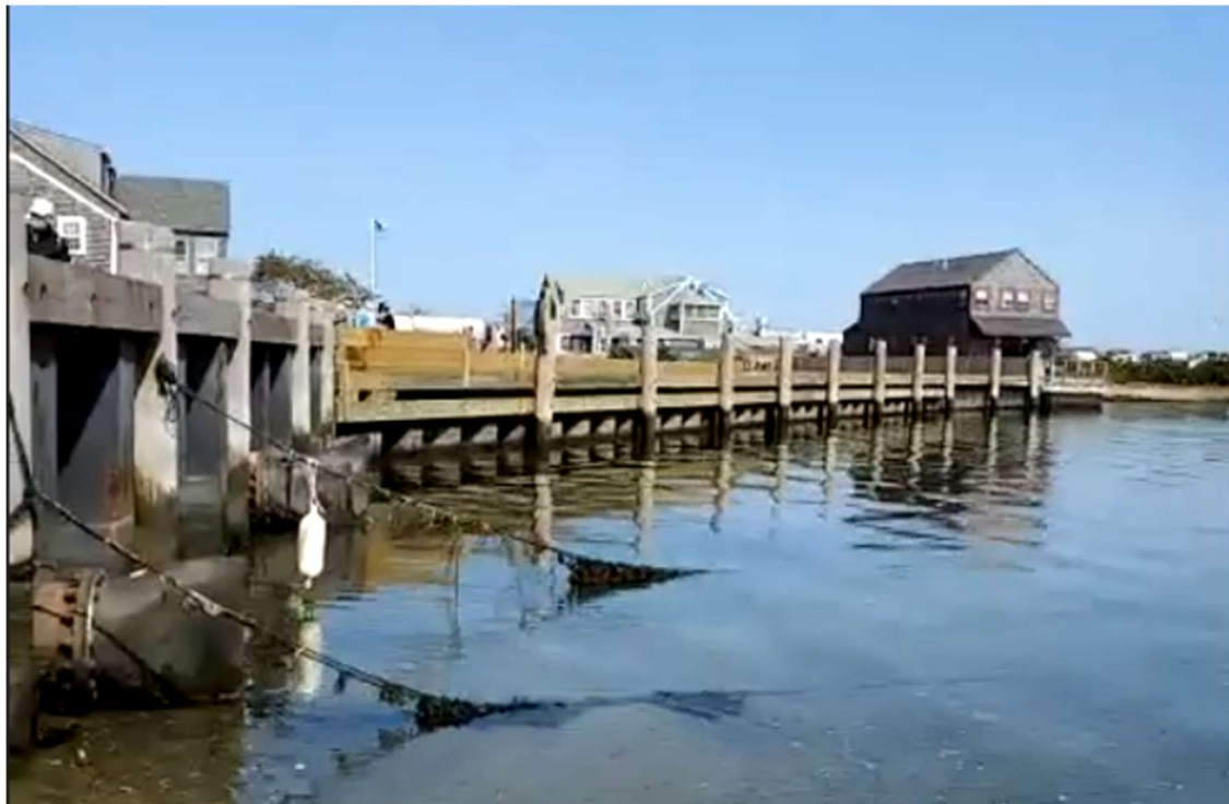
Figure 19: A wave attenuation wall near the intersection of Easy and Oak St. (V. Murphy, personal communications, Sept. 25, 2020)
