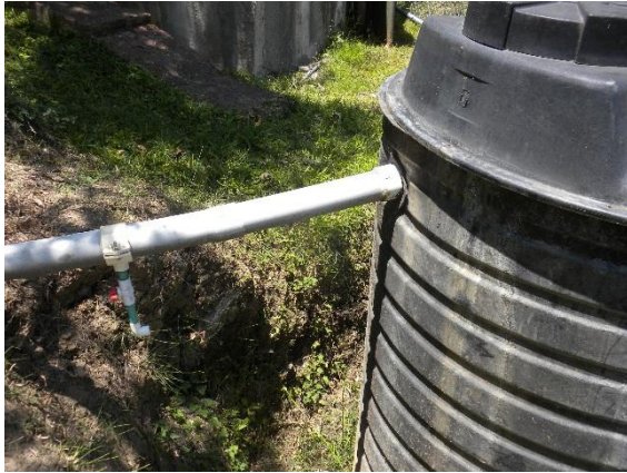
Figure 5: Ladrillera spring system test location
