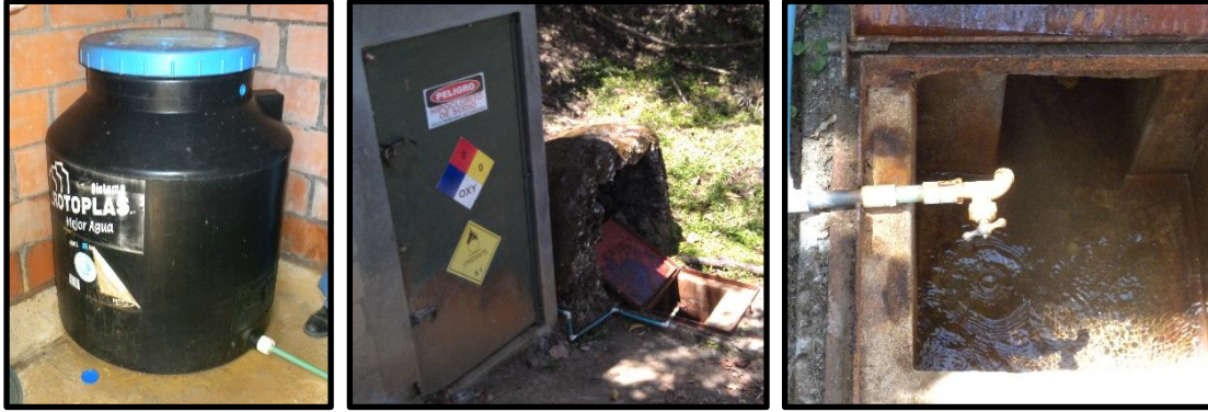
Figure 9: Ladrillera spring sodium hypochlorite disinfection system
