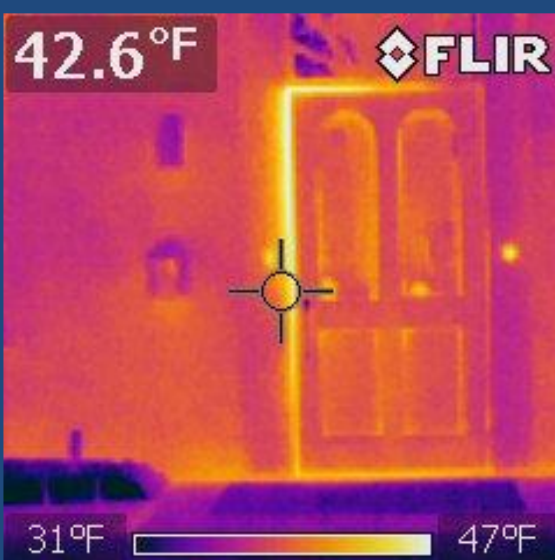
Thermal image of the front door of the Museum, showing heat loss.
