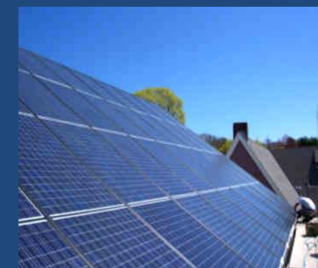
Photo-voltaic Panels on roof. ( http://www.solar design.com/projects/project_display.php?id=47 )
