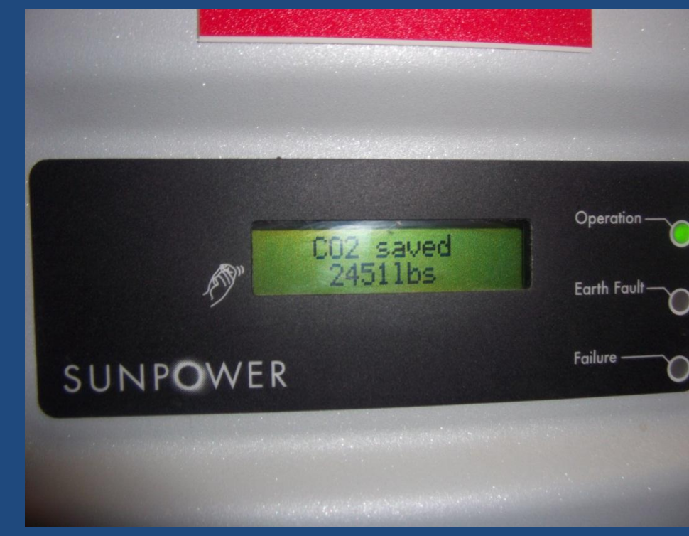
Inverter showing amount of CO 2 saved by one module
