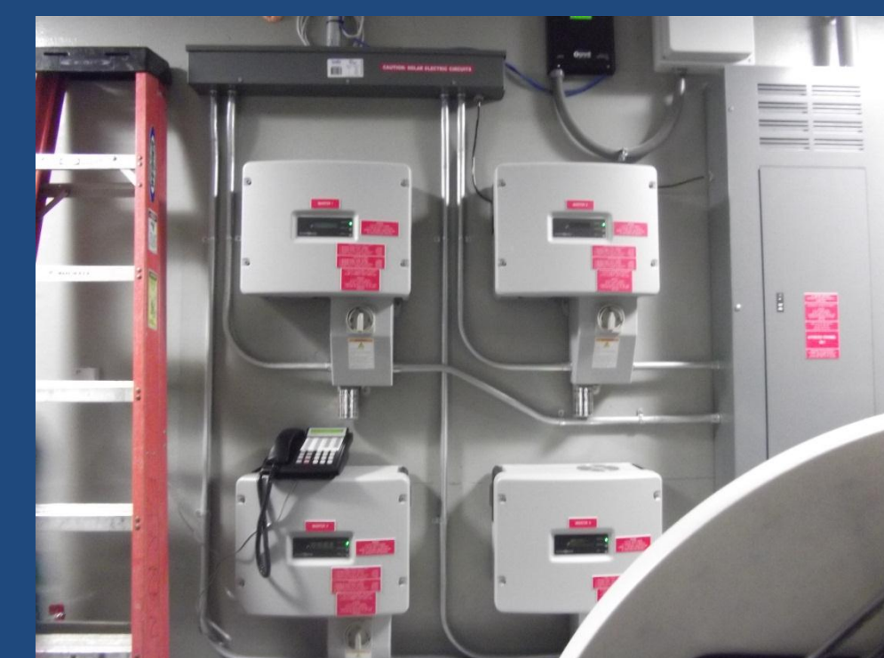
Photovoltaic Panel Inverters
