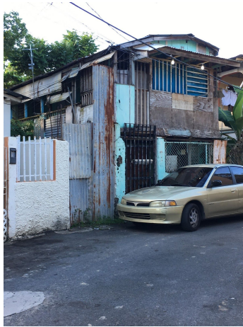
Figure 7: Example of Poor Infrastructure (2)
