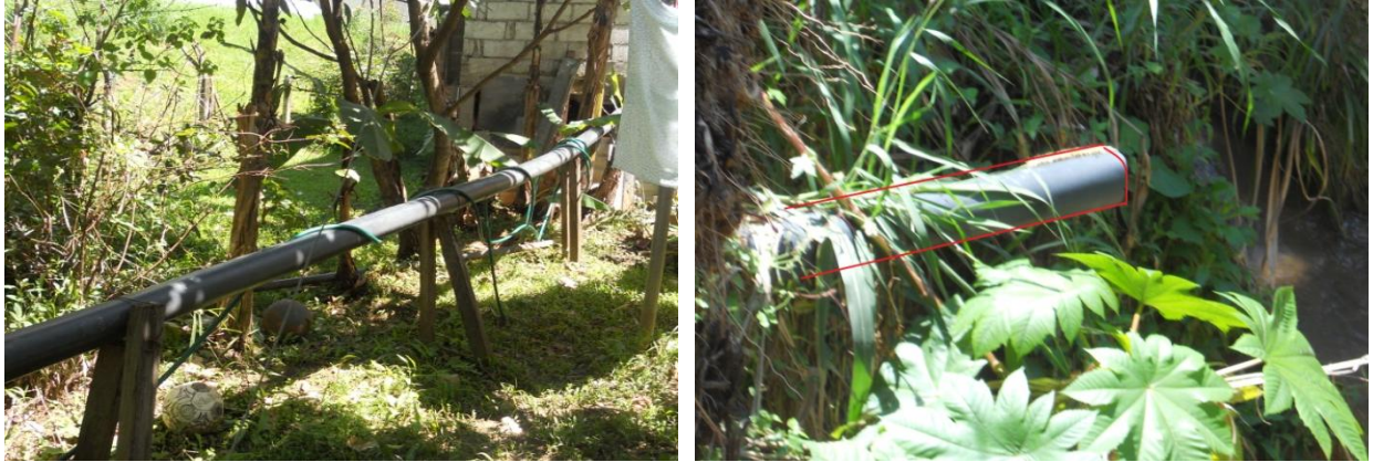
Figure 4. Current wastewater infrastructure: Pipe connecting wastewater from a house to the Quebrada Padre (left). Pipe outlet directly above the Quebrada Padre (right). (Photos by Stephany Vasquez, 2011)
