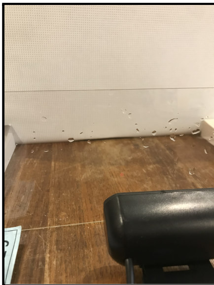
Figure 42: Water on Vertical Glass.
