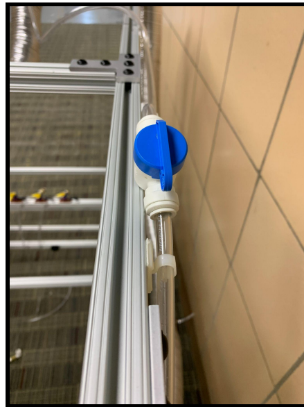
Figure 57: Valve to control Shower Head.
