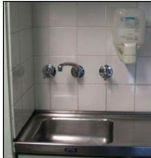
Figure 62: Corridor handwash facility
