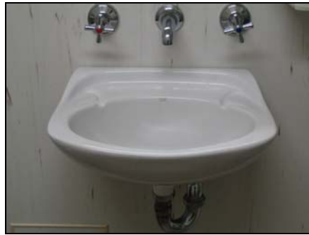
Figure 67: Central bathroom sink
