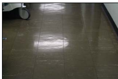
Figure 49: Glare from general flooring material used in ward
