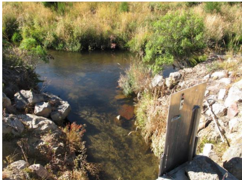
Figure 32: Unprotected intake upon arrival
