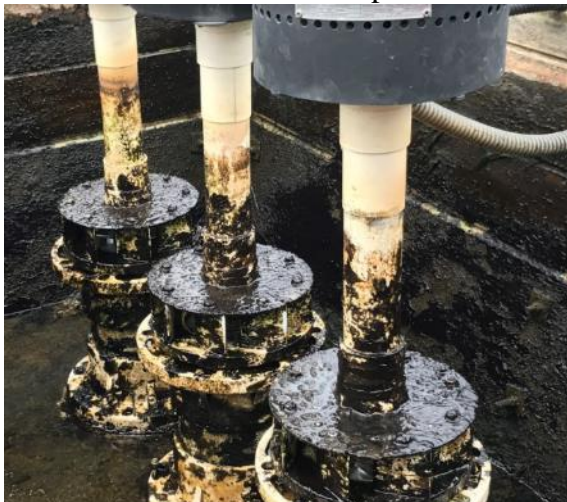
Figure 42: Turbines before cleaning
