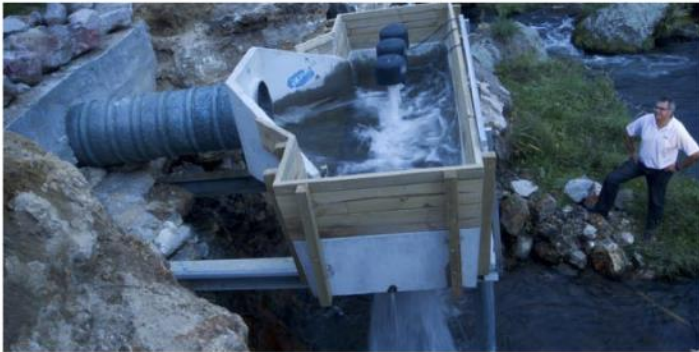
POWER BROKER: Project manager Eugene Berryman-Kamp beside the micro-hydro unit, which is saving Kearoa Marae.
