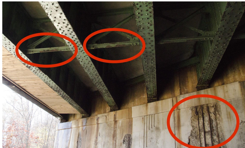
Figure 6: Corrosion and Deterioration of Existing Structure (Google Maps, 2016a).
