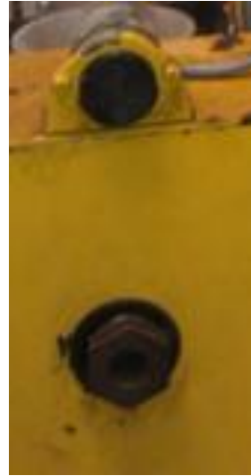
Figure 16 Missing Gasket for Speed Gage
