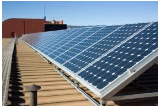
Figure 11: An example of a rooftop solar array 80
