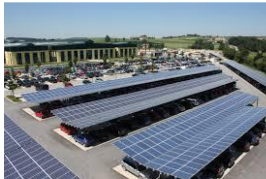
Figure 12: An example of carport solar arrays 81
