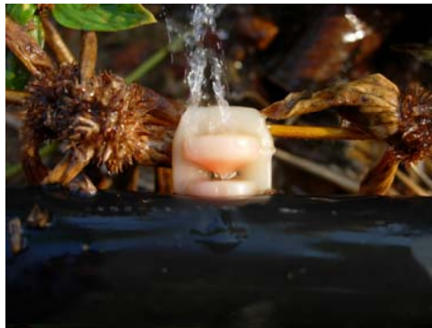
Photograph 17 : Sprinkler emitter on the lateral lines
