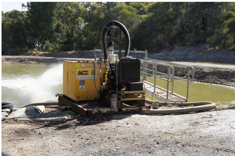
Figure 14. One of many diesel generators in operation at the Grantville facility.
