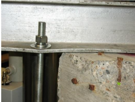
Figure 10: I-Beam Deformation in Preliminary Testing
