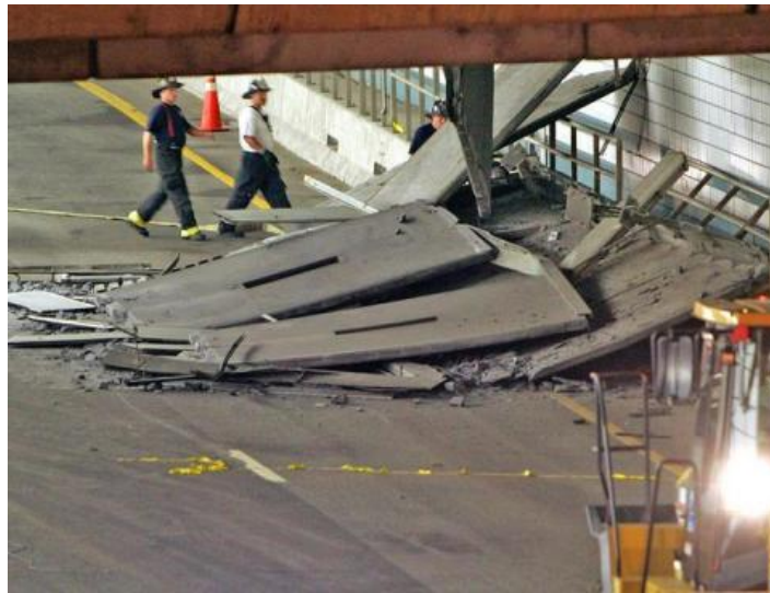
Figure 35: Big Dig Panel Collapse, news.thomasnet.com
