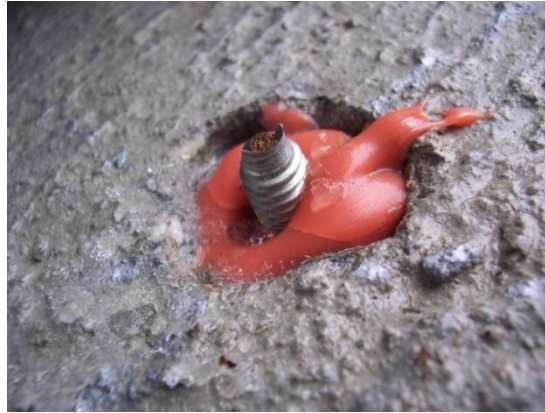
Figure 40: Cracked HIT RE 500 Adhesive
