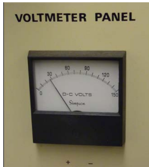
Figure 38: Voltmeter Measuring Turbine Output Voltage
