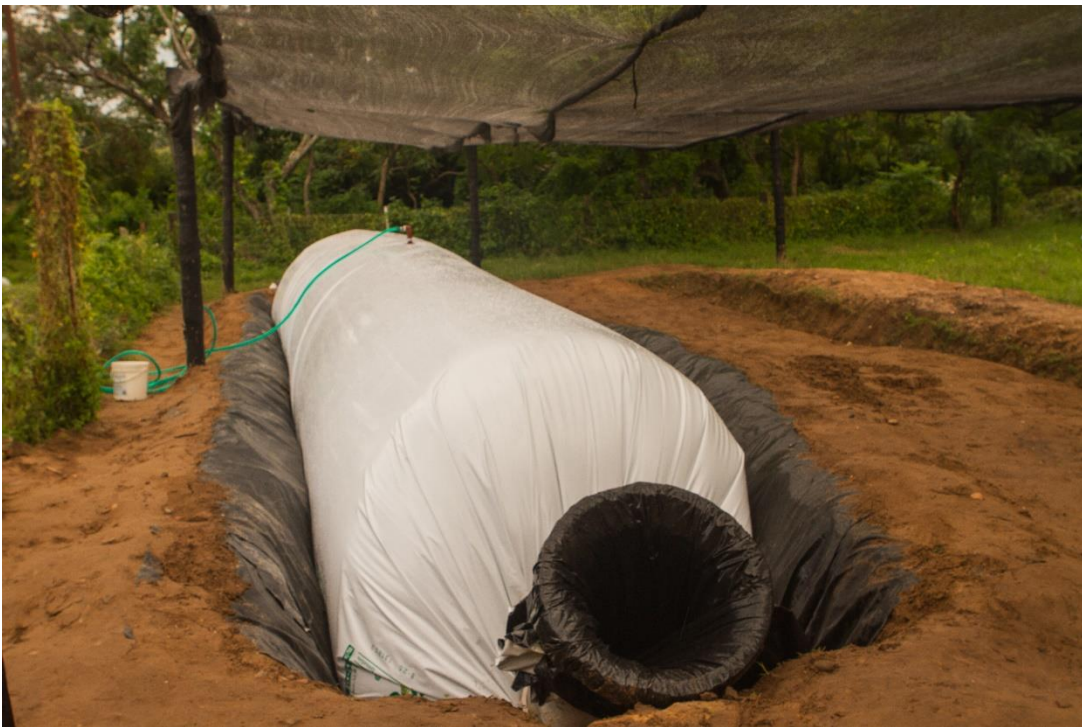
Figure 9: Lengthwise View of New Biodigester
