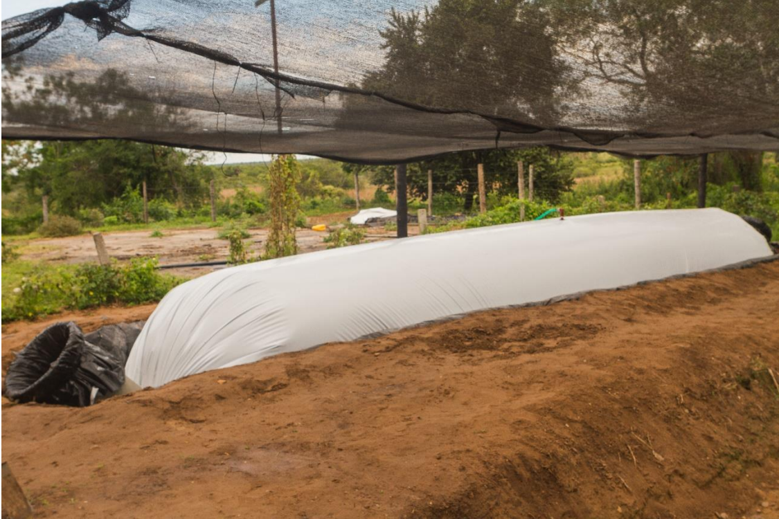
Figure 8: Horizontal View of New Biodigester
