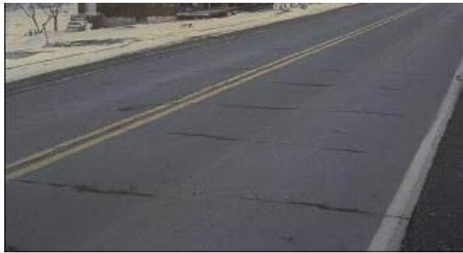
Figure 8: Transverse cracks caused by thermal cracking in a roadway pavement. 17
