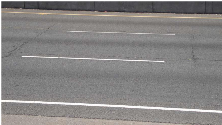
Figure 3: Reflection cracking in an HMA overlay. 10
