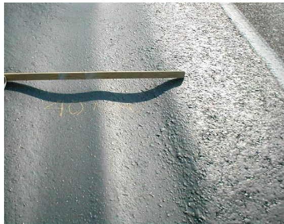
Figure 4: Rutting failure within the wheel path of an HMA pavement. 10
