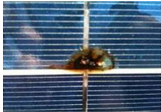
Figure 9: Module hot spot failure (First Green, 2014)
