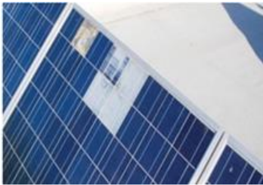
Figure 8: Module delamination failure (First Green, 2014)
