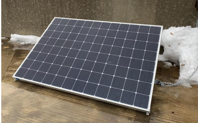
Figure 32: Mounted Solar Panel
