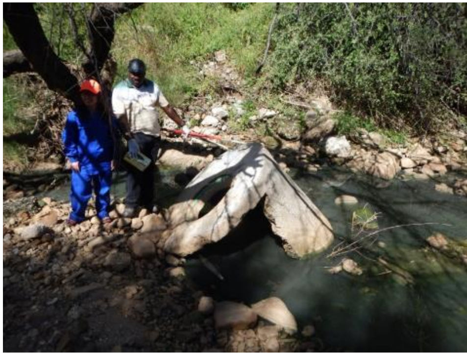
Figure 13 - Destroyed Manhole in Arebbusch River
