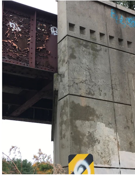
Figure 14: Existing Bridge Conditions-Map Cracking on East Side of North Abutment and Peeling Lead Paint on East Side of Girder (Hamdan, 2019)
