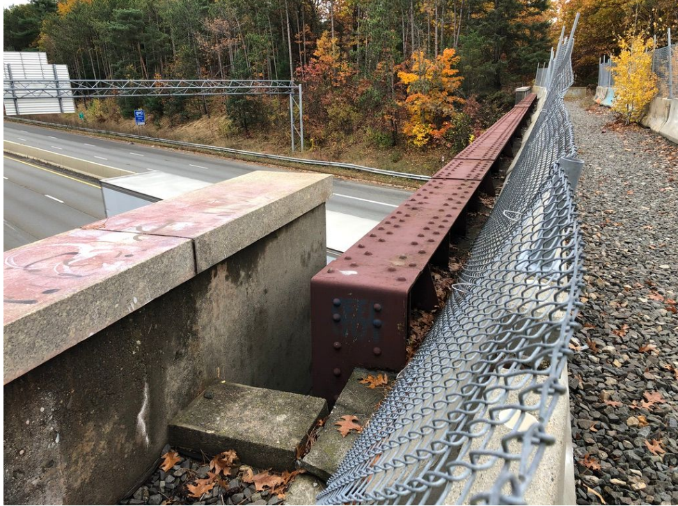
Photo 7: Looking south, collapsed bridge next to low girder, connecting to concrete abutment.
