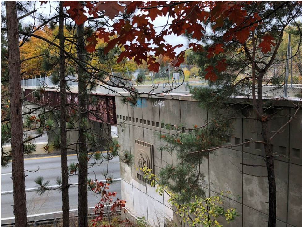
Photo 10: Looking southwest at the abutment on the north side of the bridge.
