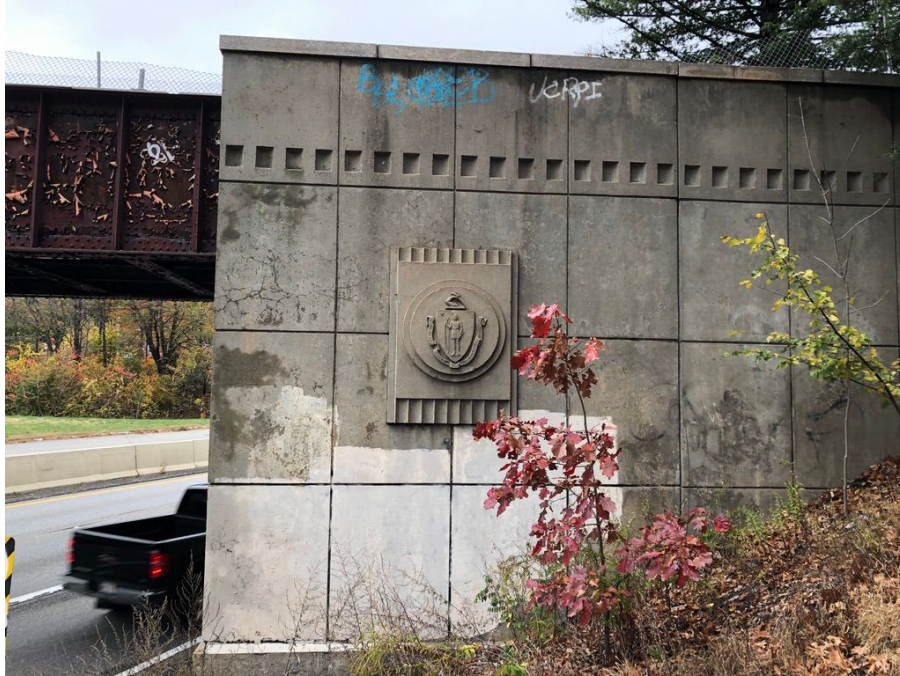
Photo 11: Looking west at the side of the north abutment of the bridge.
