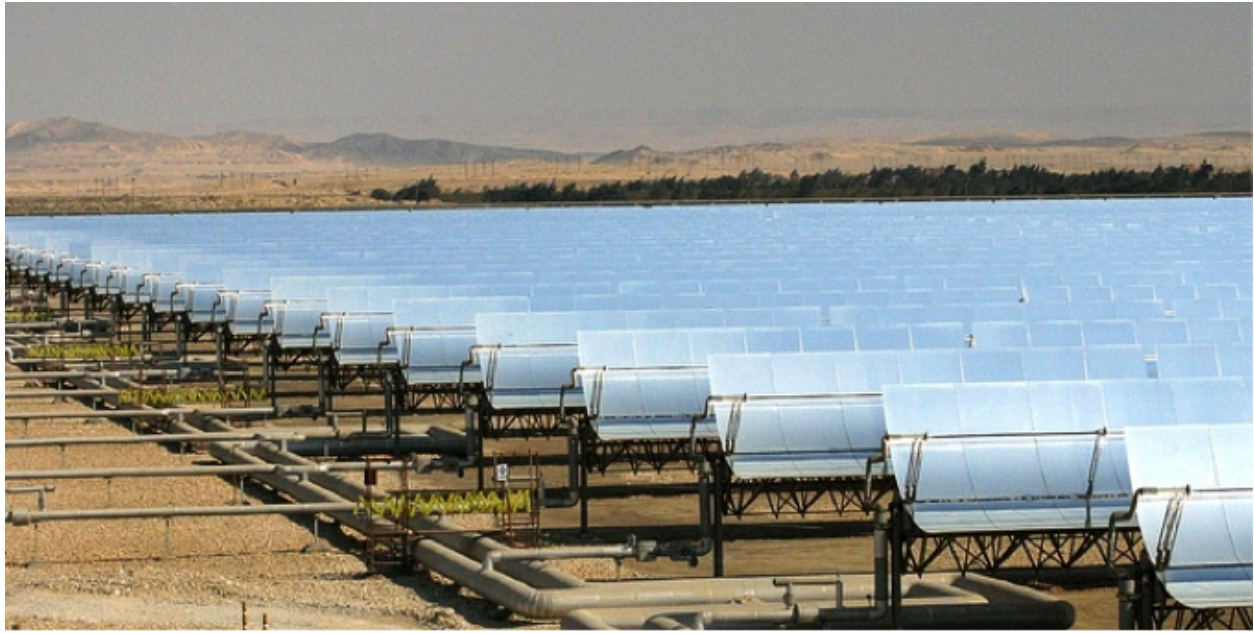
Figure 3: Kuraymat parabolic trough solar power plant
